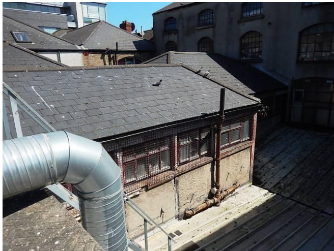
View of two-storey extension. Upper floor is used as studio space. Extension is heavily subdivided.
